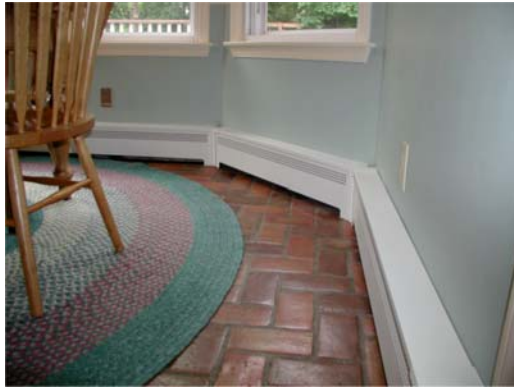
#1 – The measuring and layout for a bay window or non 90-degree corner is referenced on the Bay Window Corner Measuring Instructions and Bay Window Installation pages. Once the panels have been slipped into place, the final stage is to install the top rail wedge pieces.
