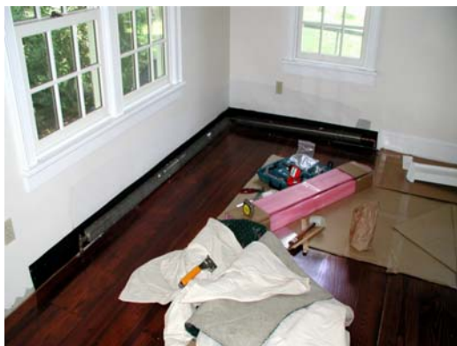
#3 – The painted tin flashing is slipped down along the wall to the floor and secured with staples, tacks, or roofing nails.
