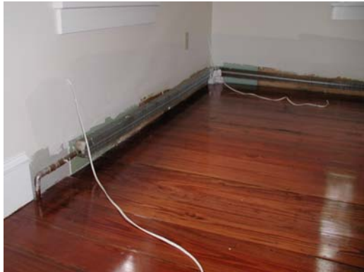
#1 – The original baseboard enclosures have been removed (see Removing Back Panel page for detail).
