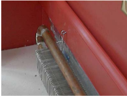
#1 – The existing support brackets for this installation were missing or removed. An eye-hook and wire assembly were used to support the plumbing and heating element.
