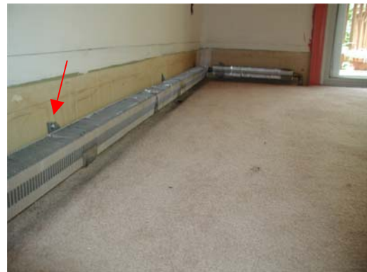
#6 – This photo shows the modified support brackets re-installed. See Re-Using Existing Support Brackets page for detail.
