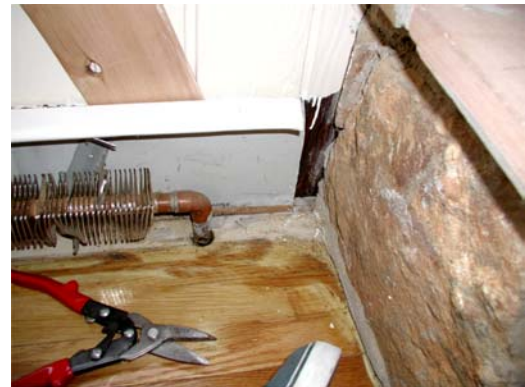
#4 – Snip out entire end section of back panel to accept new end cap or use open end caps that require a smaller notch.
