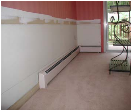
#1 – Wall area is being prepared for wainscoting installation. Existing baseboard enclosure still in place.
